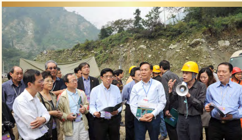
LegCo Members are briefed on the progress of the construction work of the Provincial Road 303 Yingxiu to Wolong section.
