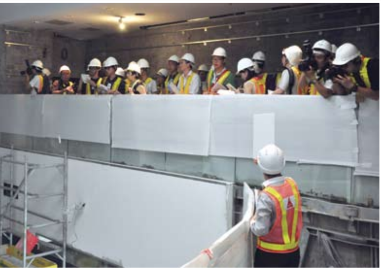
Media representatives tour the Complex to learn more about the progress of the construction work and the facilities and services to be provided in future.
