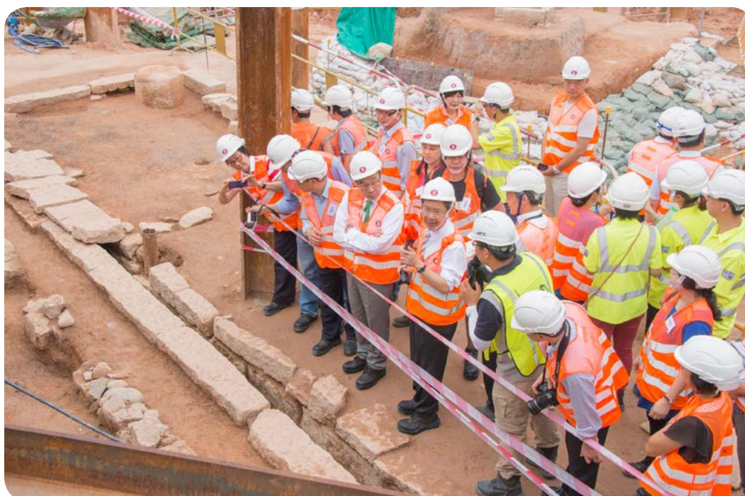
Members of the Panel on Transport at the construction site of the To Kwa Wan Station of the Shatin to Central Link.
