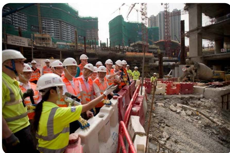
Members of the Subcommittee on Matters Relating to Railways at the construction site of the West Kowloon Terminus of the Hong Kong Section of the Guangzhou-Shenzhen-Hong Kong Express Rail Link.
