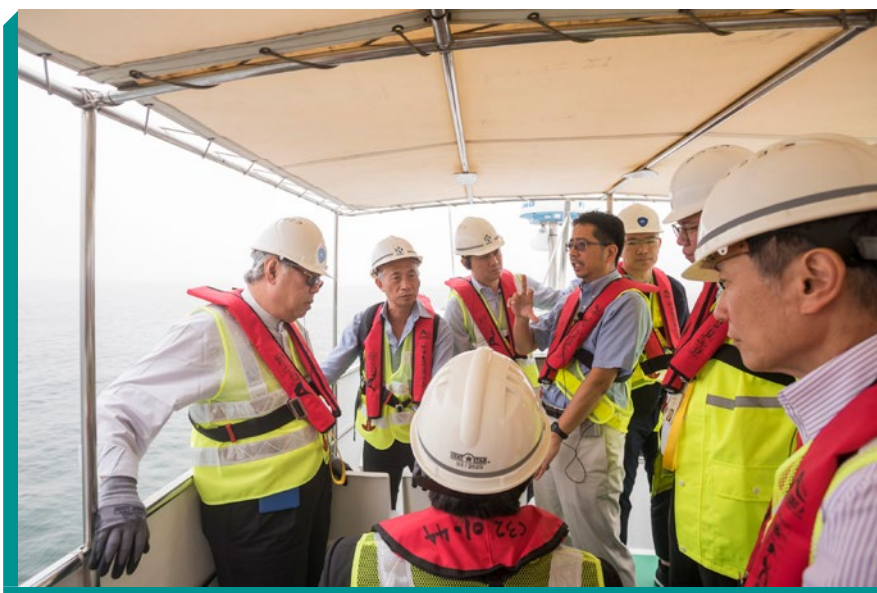
Members of the Subcommittee to Follow Up Issues Relating to the Three-runway System ("3RS") at the Hong Kong International Airport take a boat trip to observe the 3RS reclamation works area.
