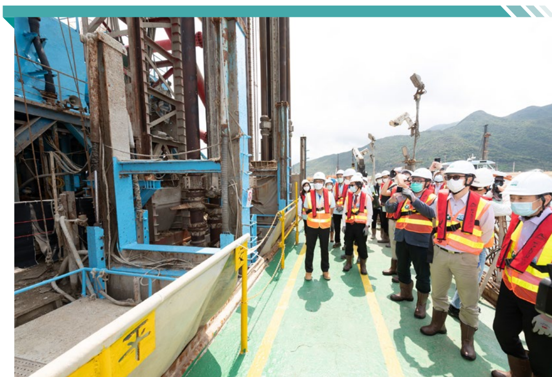
Panel members observe the operation of the non-dredge ground treatment method of Deep Cement Mixing
