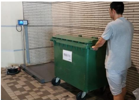
Waste weighing system to record the daily waste quantity
