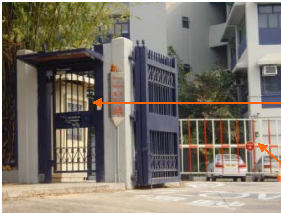
Automated Security System
