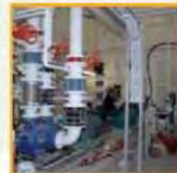
Sprinkler fixed & fire services booster pump room
