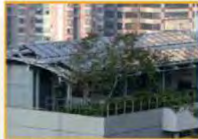
Rooftop solar photovoltaic panels can convert solar energy to electrical energy for the building
