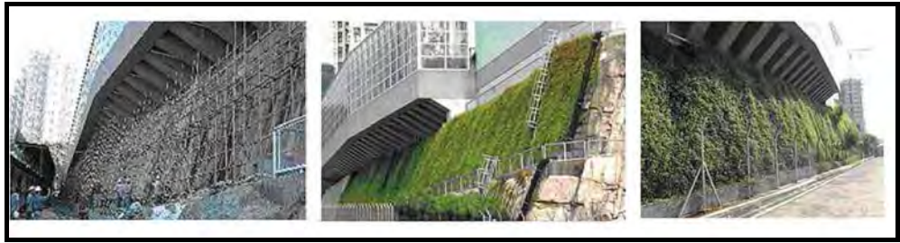
Proprietary mulching method trial at the man-made slope in Yau Lai Estate Phase 1
