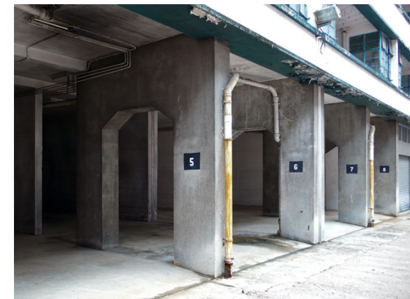
支柱強調了房屋與地面的接觸形態 Articulation of ground contact with supporting elements
