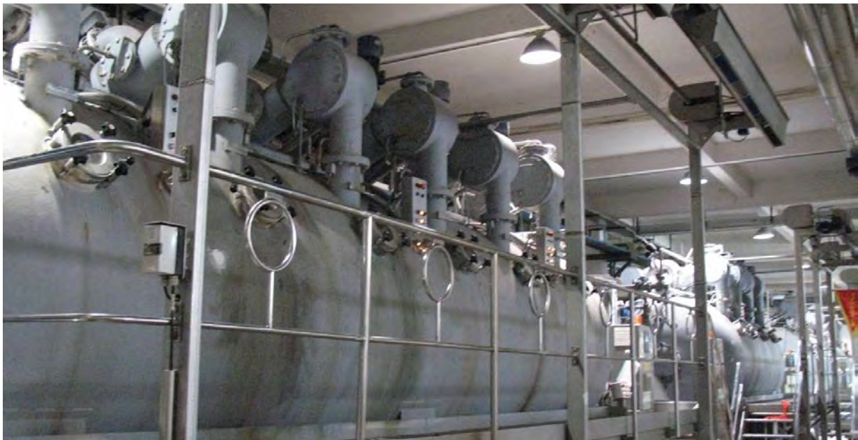
Figure 3-5 “Cleaner Production Partnership Programme” demonstration project– energy efficient dyeing tank with thermal insulation: as of end July 2011, the CPPP subsidized 1,469 projects. The Programme, which was jointly launched by Guangdong and Hong Kong, facilitates enterprises to conserve energy, reduce emissions and enhance cost-effectiveness.
