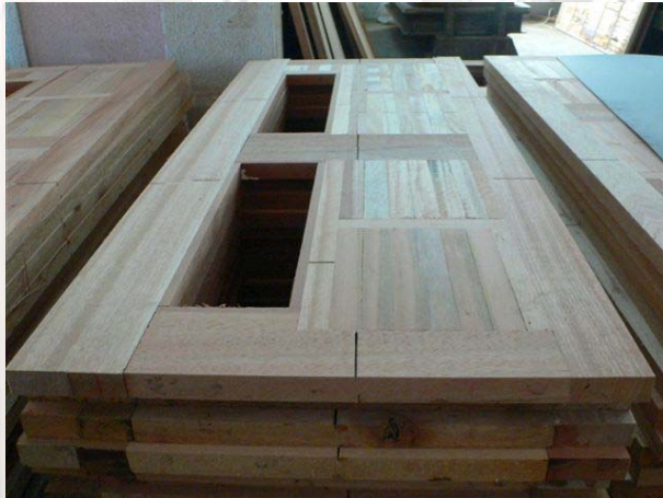
(5) Core Assembly Completed
