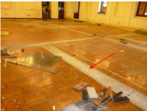
The square-patterned timber strip flooring finish reviewed after the removal of carpets. Trunk damages are discovered. (pointed)
