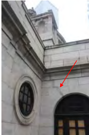
Fig. 23 Cracks developed on various locations on the building which led to the temporary closure of the entire building in 1978 for restoration. The photo shows one of the cracks located on the granite surface in 2/F under the central dome being repaired in 1980s. (Pointed)
