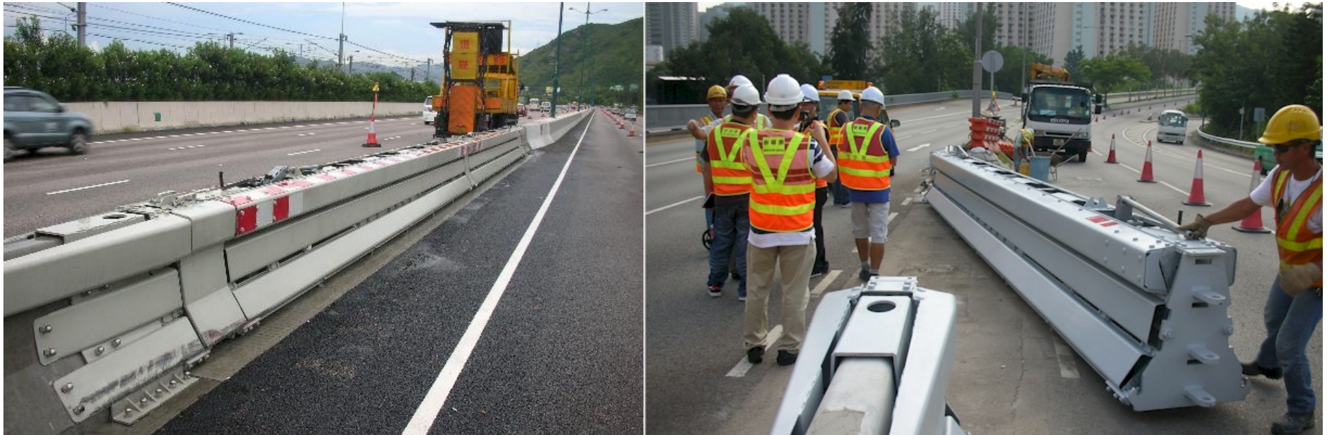
Figure 2: Movable Steel Barriers
