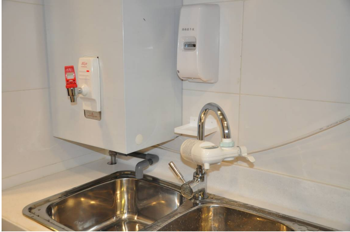
Filters have been installed on the water taps in the pantries of the LegCo Complex.
