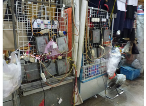
Figure 2.6.2 - Improper /Overload Connections of Power Supplies
