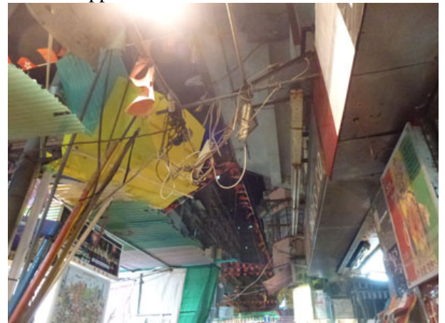
Figure 2.6.3 - Illegal Connections of Power Supplies
