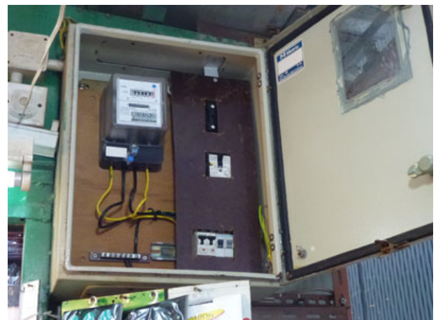
Figure 3.8.3 – Internal Layout of Power Distribution Box
