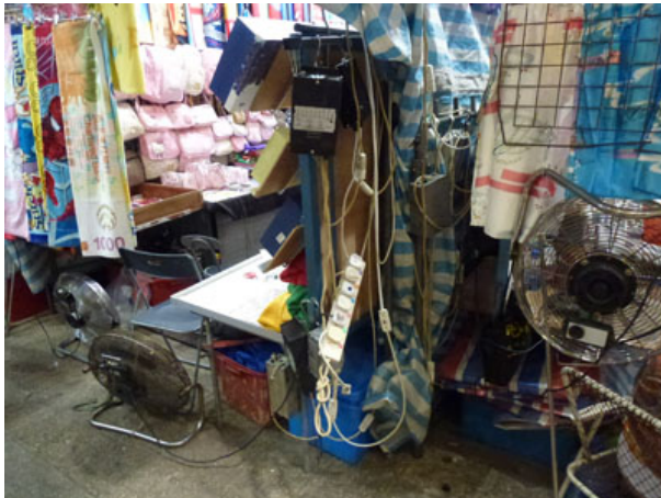
Figure 2.6.5 – Improper / Overload Connections of Power Supplies
