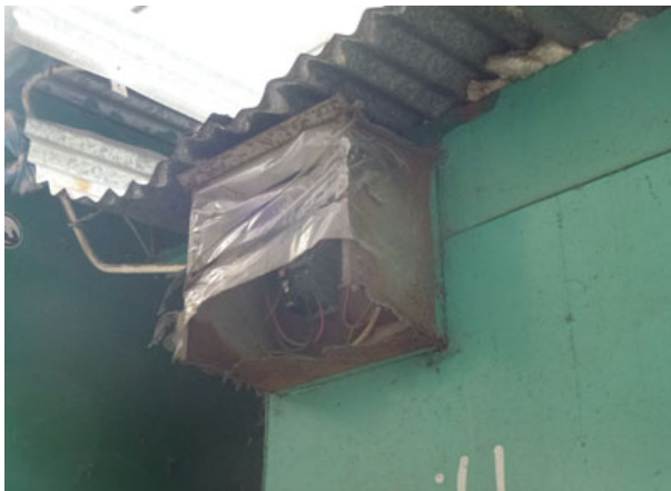
Figure 2.6.1 - Damaged Power Box Lack of Maintenance
