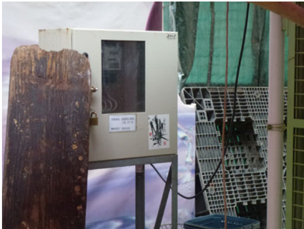
Figure 3.8.5 – Free Standing Power Distribution Box
