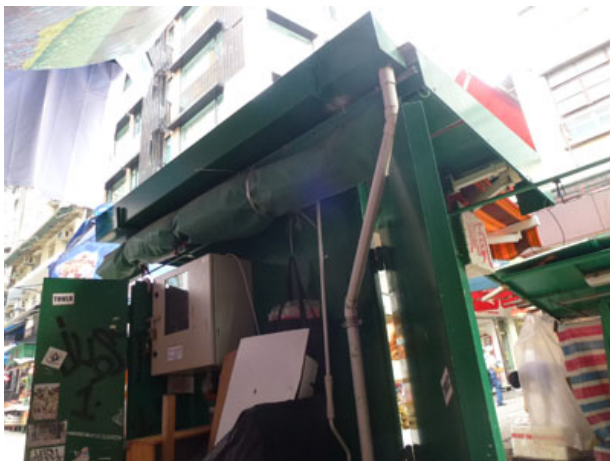
Figure 3.10.1 – Rain Water Collection System of Hawker Stall
