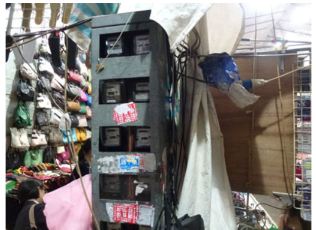
Figure 3.8.8 – Broken Power Pillar at Tung Choi Street
