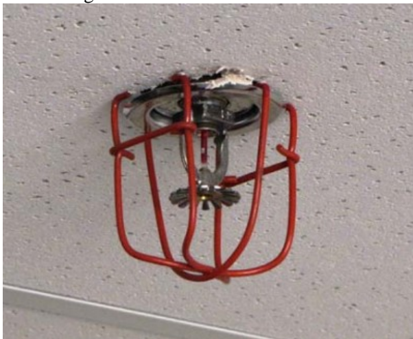
Figure 7.5.2 – Protective Guard for Sprinkler Head
