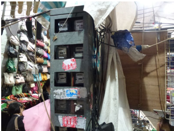
Figure 2.6.6 – Damaged Power Box and Illegal /Substandard Connections of Power Supplies
