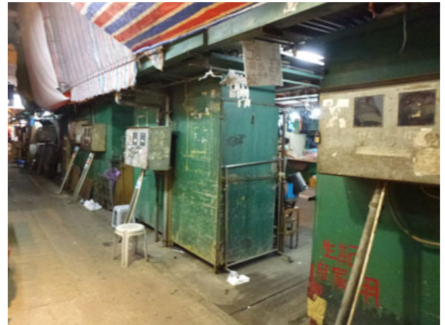
Figure 3.8.2 – Large Power Distribution Boxes for Two Hawker Stalls
