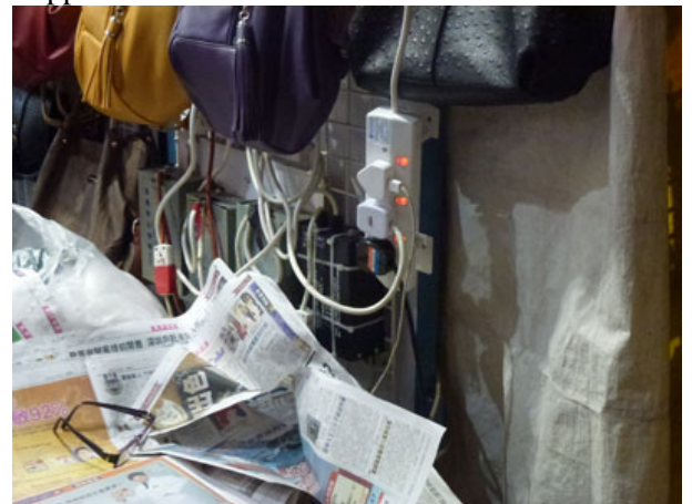
Figure 2.6.4 - Overloaded Power Points Covered by Combustibles
