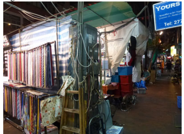
Figure 3.8.7 – Power Pillar at Temple Street with Cables in Mesh
