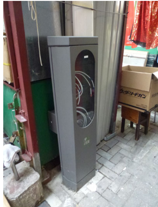
Figure 3.8.6 – Power Pillar at Tai Yuen Street
