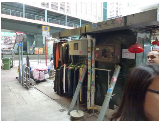
Figure 3.8.1 – Power Distribution Boxes with Tilted Cable Conduits
