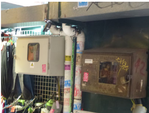
Figure 3.10.2 – 100 mm diameter Rain Water Pipes
