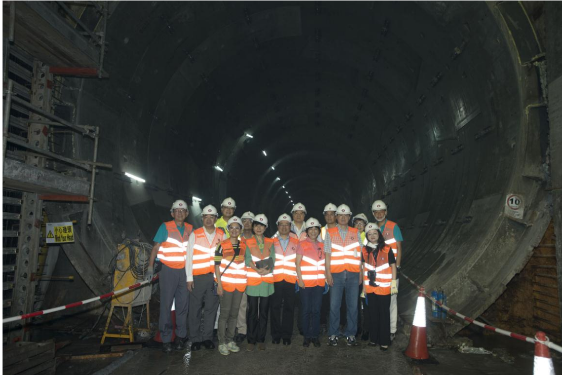
LegCo Members visit the site of main tunnel of the XRL and take a group photo with the representatives of the MTR Corporation Limited.
