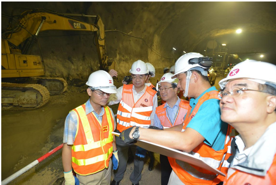
LegCo Members receive a briefing from a representative of the MTR Corporation Limited on the construction works during their visit to the main tunnel of the XRL.
