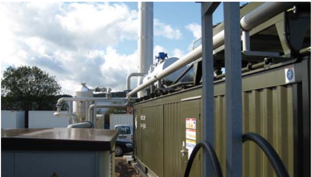
A cogeneration unit for energy production at an anaerobic digestion plant
