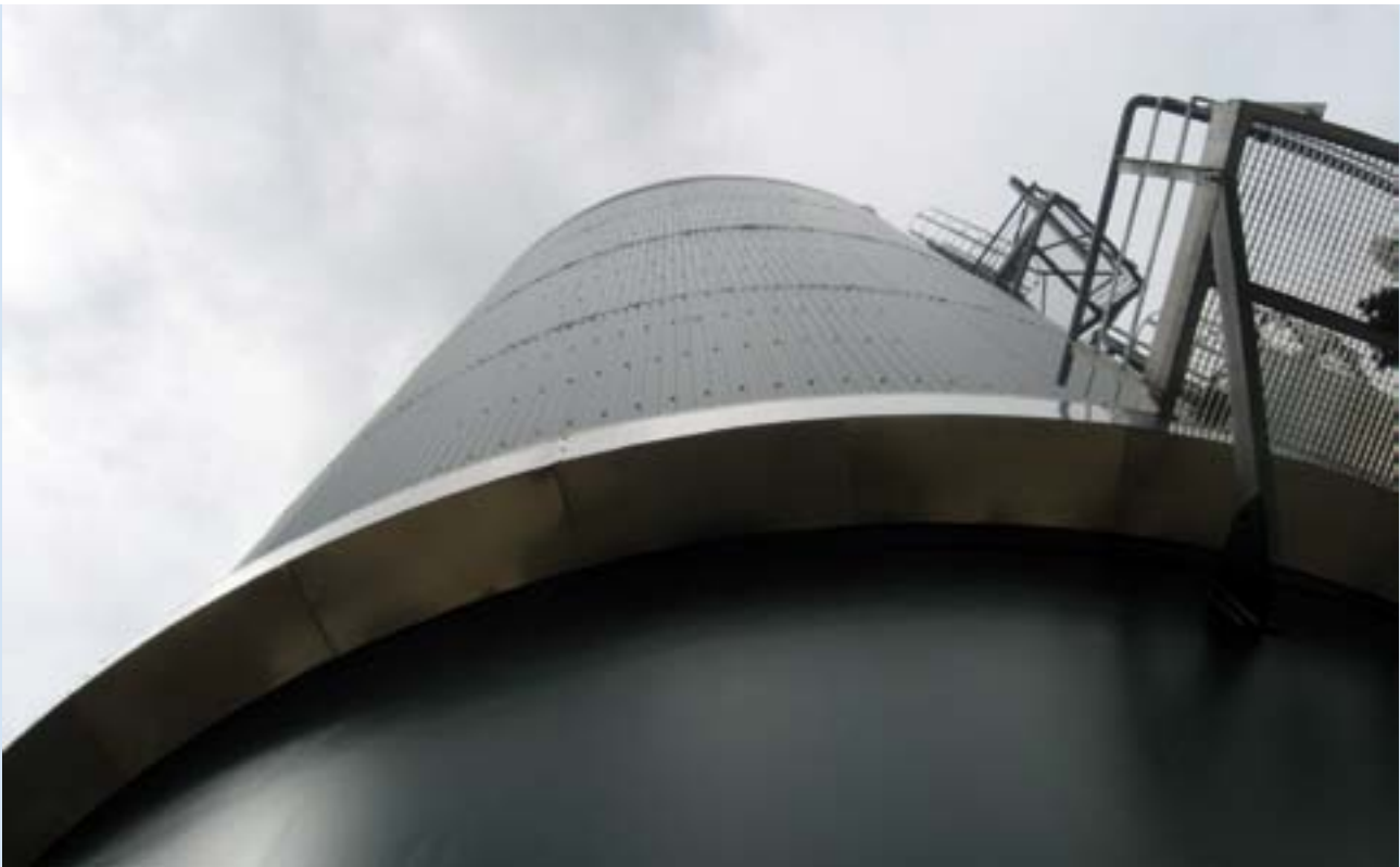
Digester of a biogas facility
