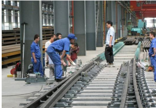
與信號系統進行道岔功能測試 Turnout Functional Test with Signalling System
