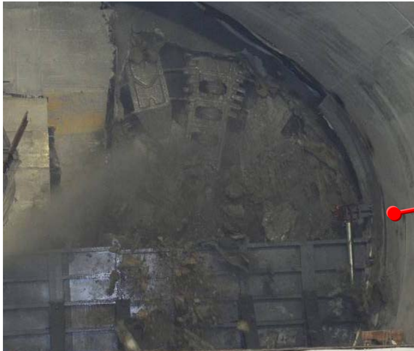
南昌以北的北行隧道於2013年11月貫通 Breakthrough of up-track tunnel at the north of Nam Cheong in Nov 2013
