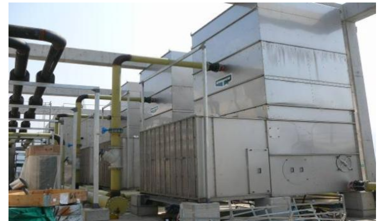
石崗大樓之冷卻水塔 Cooling Tower at Shek Kong Main Building
