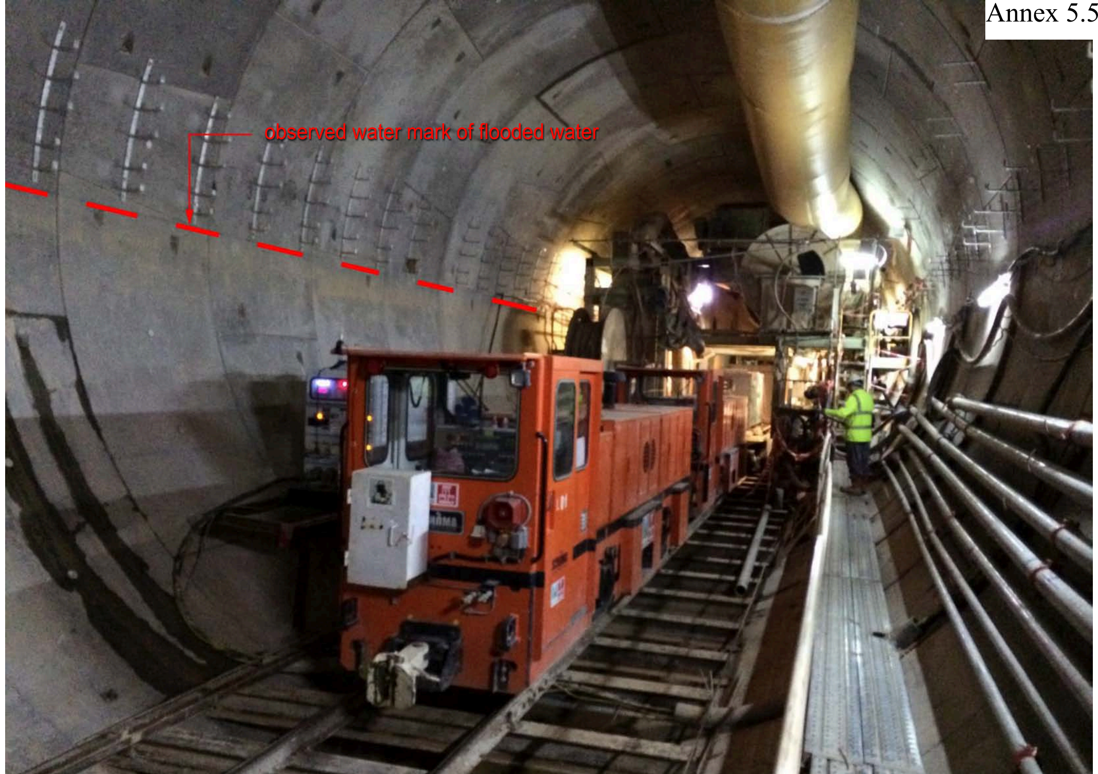
Photo showing the water mark left behind within the flooded tunnels
