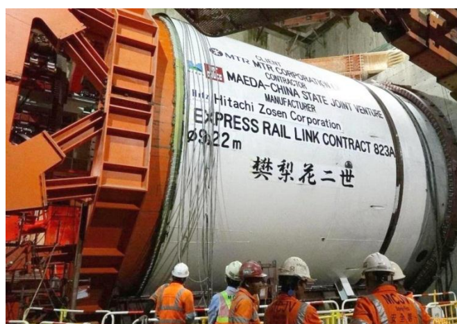
The second TBM was launched in March 2013 to catch up with delays in the Yuen Long tunnel section.
