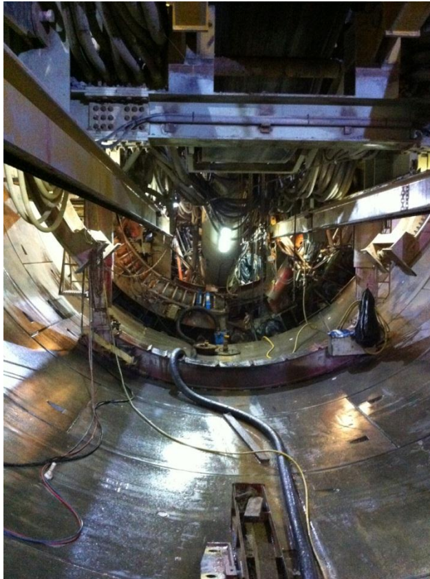
The flooded TBM with damaged components inside the Yuen Long tunnel.
