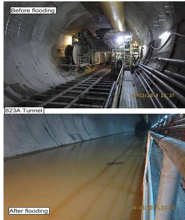
Flooded TBM tunnel
