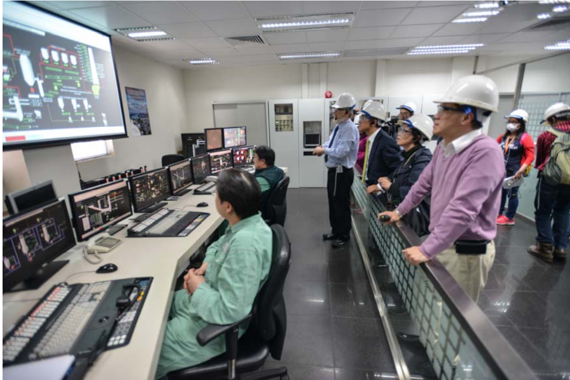
Legislative Council Members visit the central control room at the Chemical Waste Treatment Centre in Tsing Yi to learn about the operation and treatment processes of the Centre.
