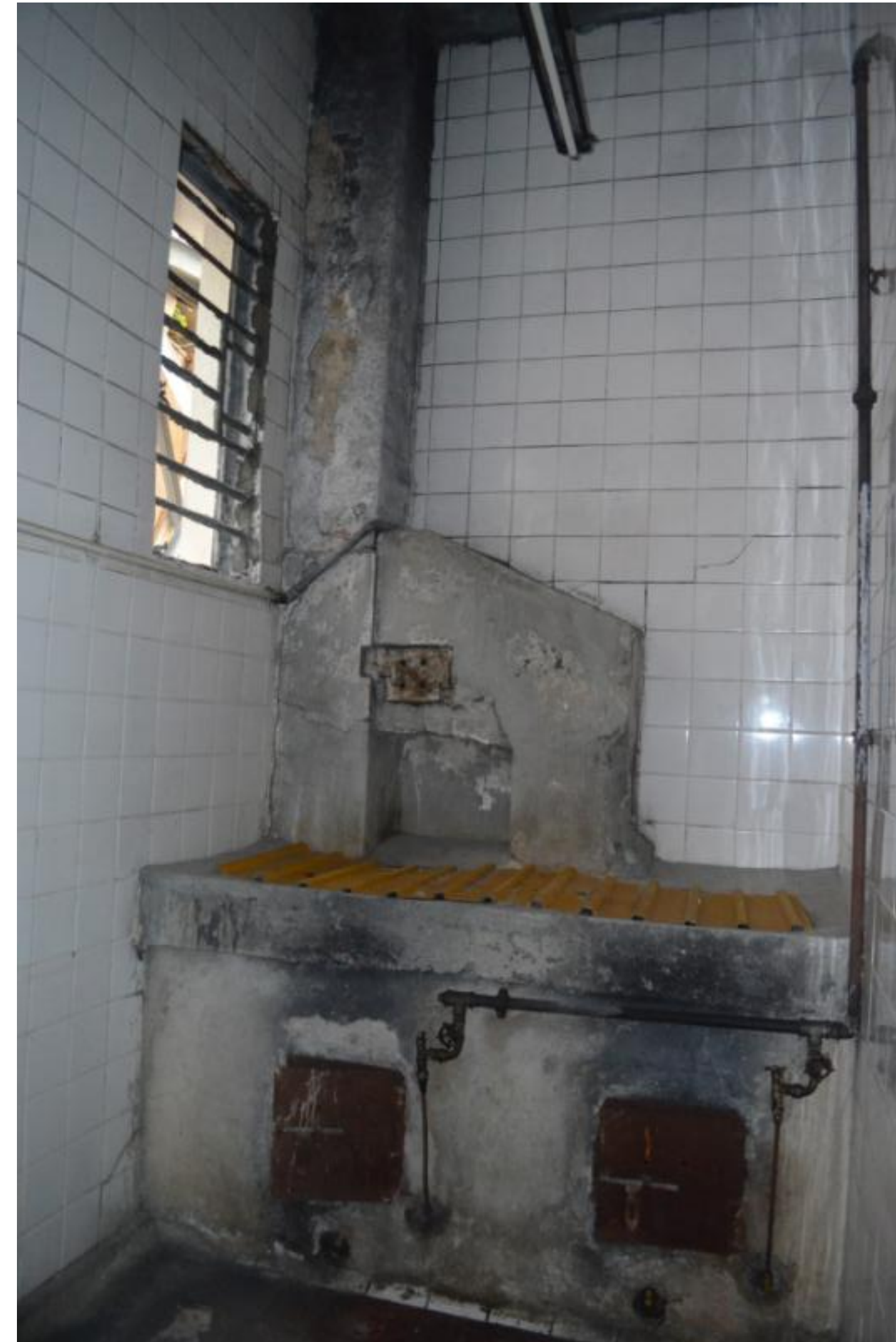
Stoves in poultry scalding room 家禽屠宰房內的爐具和煙囪
