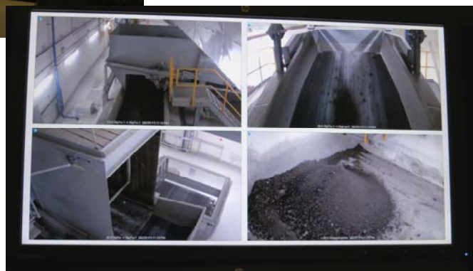
The control room of KARA/NOVEREN's Waste-to-Energy Facility where staff will monitor the waste-to-energy process 24 hours a day
