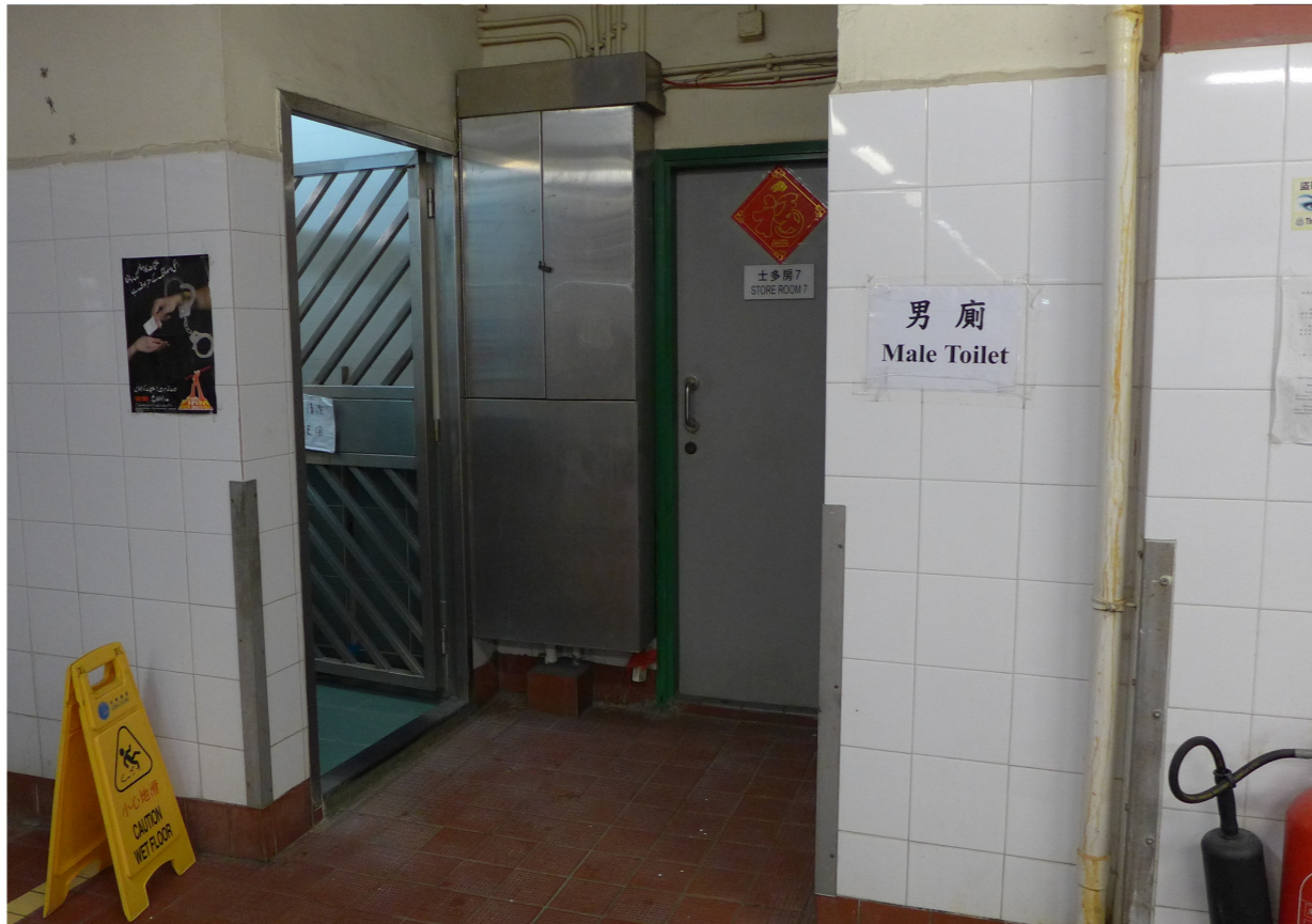
TOILET CONDITIONS ARE DIMMED AND SMELLY
