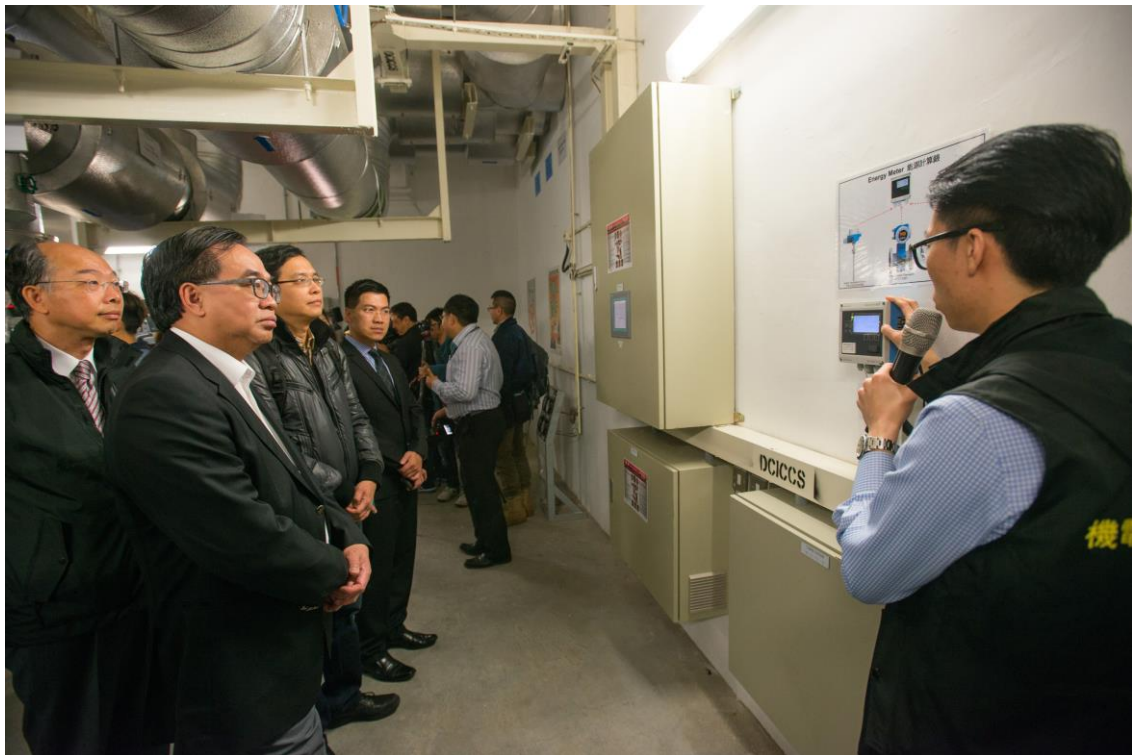
Legislative Council Members observe the district cooling system substation of the Ching Long Shopping Centre.
