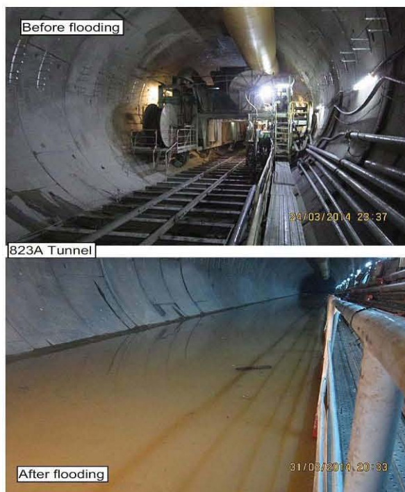
Flooded TBM tunnel
