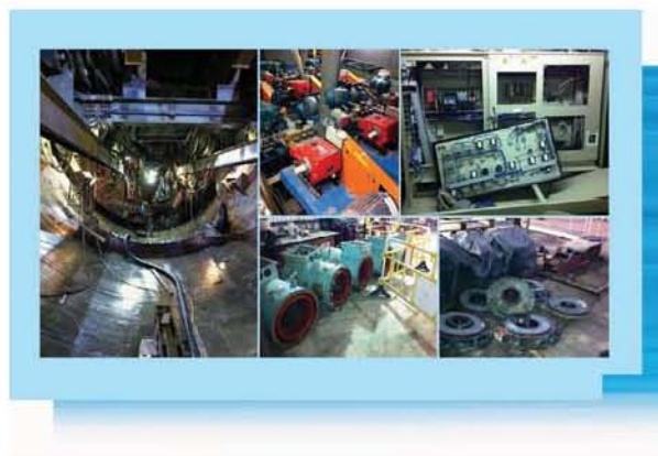
Damaged TBM at contract 823A
