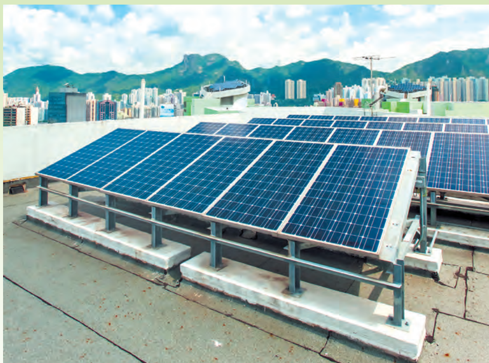
■ A grid-connected PV system.
