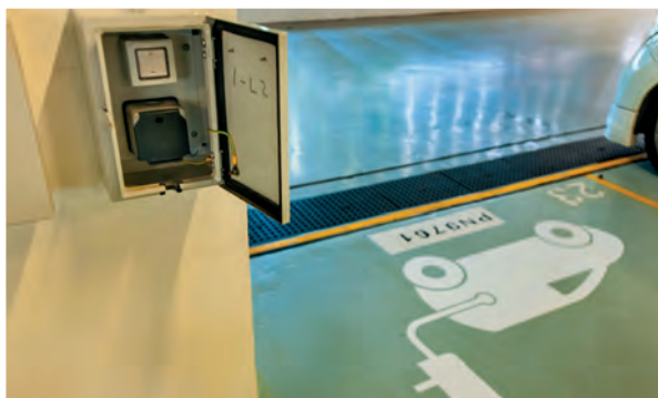
■ An EV charging facility in the Cheung Sha Wan Estate carpark.
