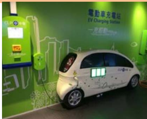
電動車輛充電設施 Electric vehicle charging facilities
