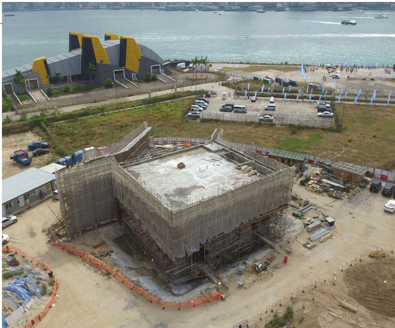
Overall view – Completion of the building structure construction 整體外觀 – 大樓結構竣工
