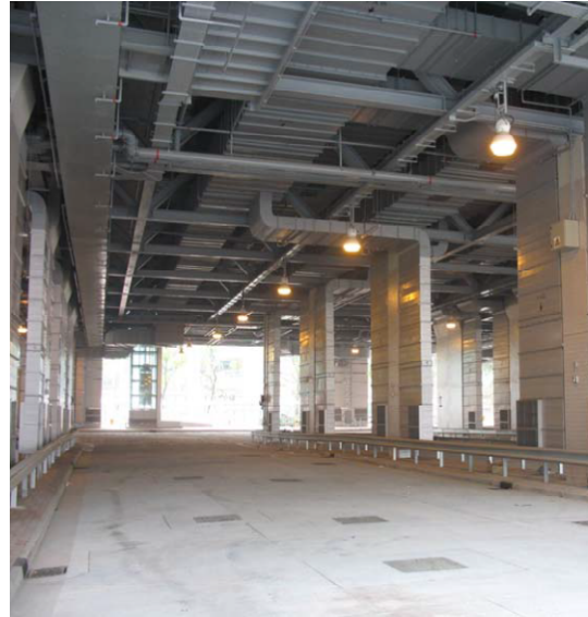
(f) High bay lights at a public transport interchange
