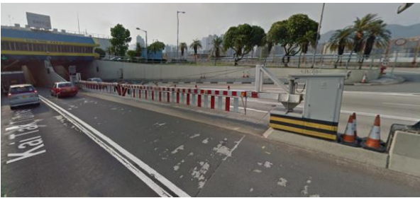
Existing movable barrier gates at the tunnel entrances could incur severe injuries if an errant vehicle collides with the equipment. The Project should specify passive safety requirements to contemporary standard for the replacement.
