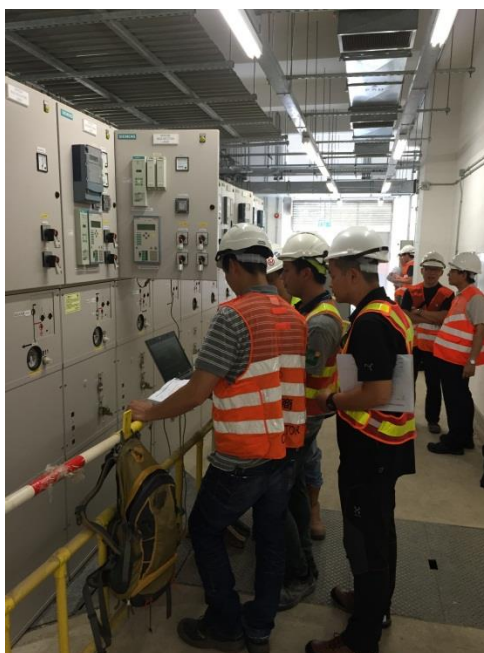
Inspection for the 25kV overhead line energisation at the Running Maintenance Shed at Shek Kong
