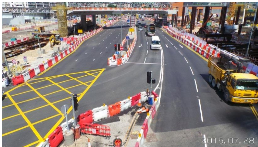
Reinstatement of Jordan Road to its permanent location was completed in July 2015
