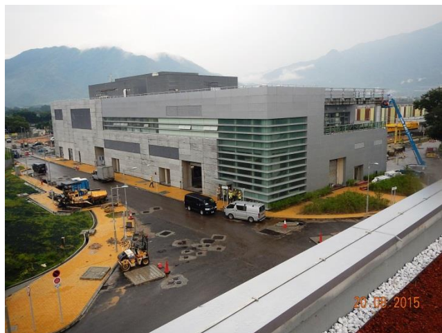
Main Building at Shek Kong Stabling Sidings (SSS) and Emergency Rescue Siding (ERS)
