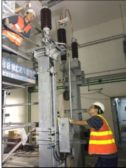
Resistance test for the jumper cable with the infeed isolator in Mongkok West Ventilation Building
