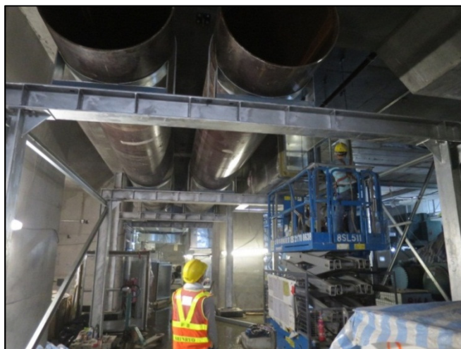
Installation of condensing water pipe header at Chiller Plant Room in WKT
