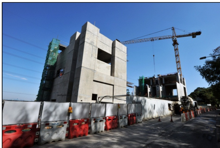
General view of the Ngau Tam Mei Ventilation Building in Yuen Long
