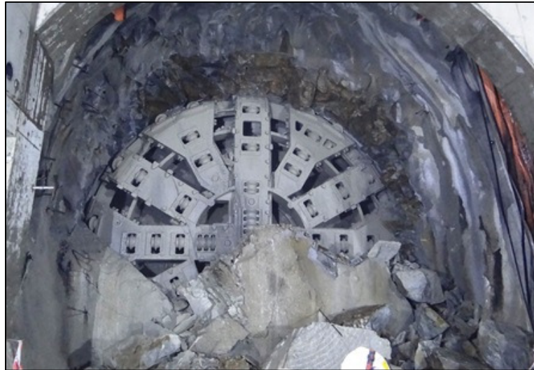
Breaking through of the northern northbound track tunnel from Tai Kong Po to Tse Uk Tsuen under Contract 823A marked the completion of excavation of the entire XRL tunnel system
