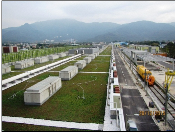
Green roof of the Running Maintenance Shed at Shek Kong Stabling Sidings (SSS) and Emergency Rescue Siding (ERS)
