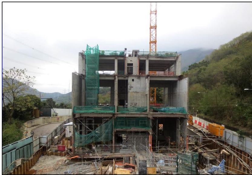
The Ngau Tam Mei Ventilation Building in Yuen Long is taking shape.
