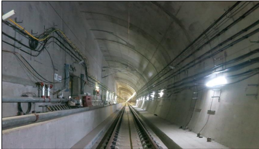
Trackside E&M installation works at southbound tunnel from Shek Yam to Mei Lai Road
