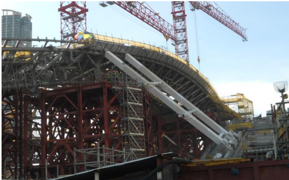
Secondary and tertiary steel members to be erected at the eastern side of the Station Entrance Building
