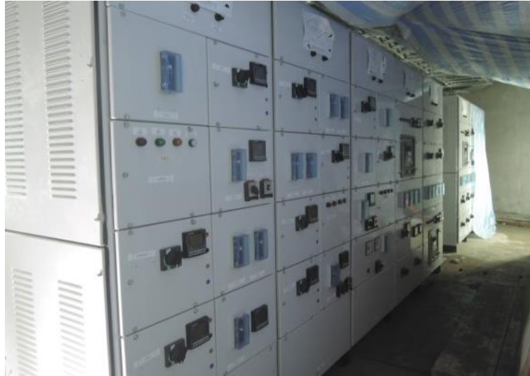
Main LV Switchboards at WKT Level B3
