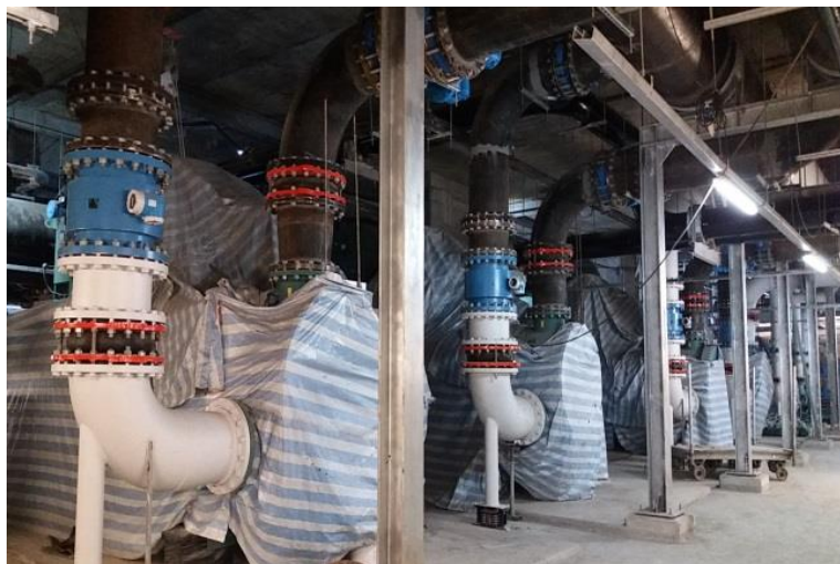
Installation of the central chiller plant at WKT Level B3 is substantially complete
