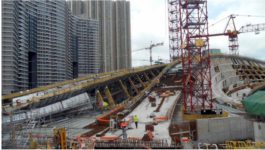
Concreting of roof trusses at the northern side of the Station Entrance Building
