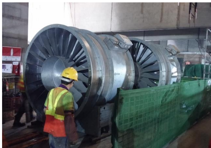
Ventilation fans are delivered to the platform level at WKT
