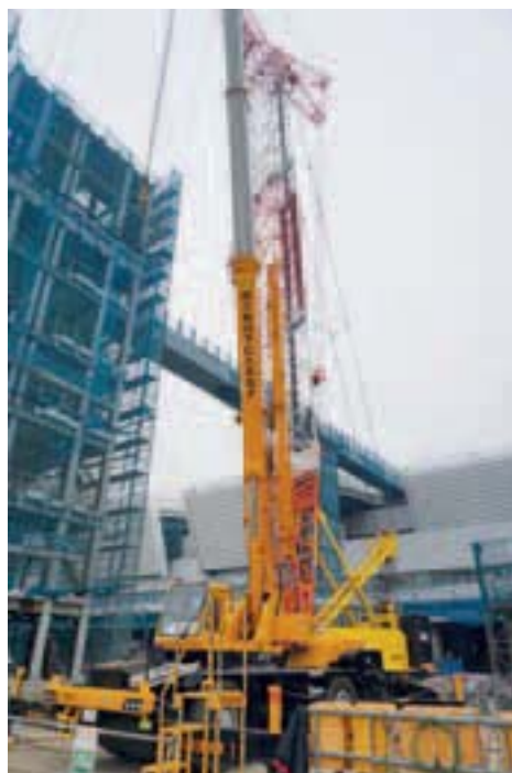
考察團參觀正在興建的日本新築地市場旗艦工程，機會難能可貴。 The delegation had the rare opportunity to visit the new Tsukiji Market, a flagship project currently under construction in Japan.
