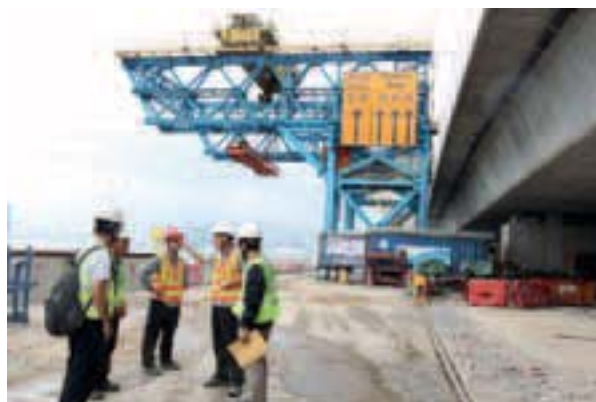
建造業乃高風險的行業，業界對相關課程特別是「安全施工程序」及「危害識別活動」需求愈趨殷切，課程可有效提升學員預防工地危害的能力。 Construction is a high risk industry. The industry has an increasing demand for related courses especially “Safe Working Cycle” and “Hazard Identification Activity” courses. These courses can effectively equip trainees to reduce potential hazards on site.
