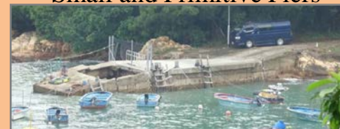
破舊碼頭 (由村民興建) Dilapidated Piers (built by locals)
