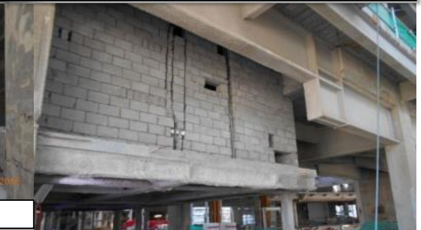
Blockworks and mechanical, electrical and plumbing (MEP) works 磚牆、機電及管道工程
