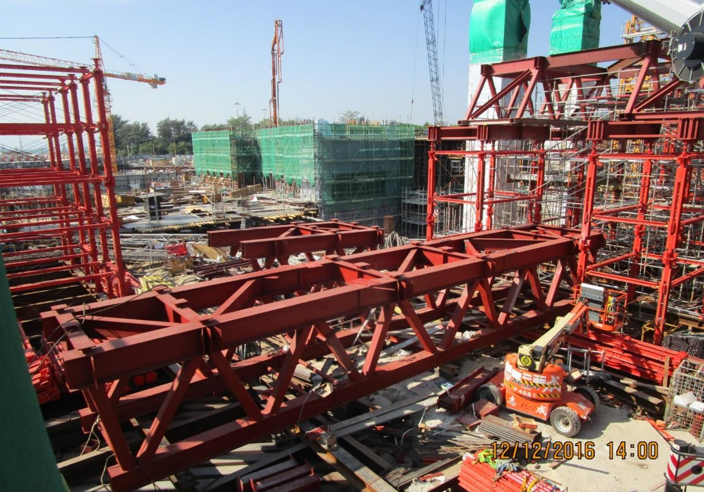
Assembly of 18m Temporary Truss for Trusses 1 & 2 為搭建第一及二號桁架而裝配十八米長的臨時桁架
