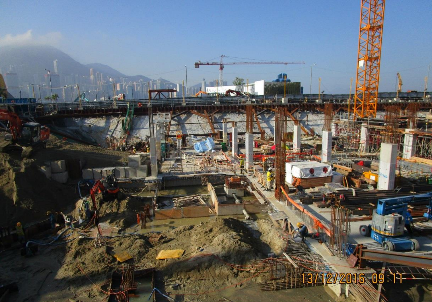
Excavation and Lateral Support (ELS) Stage 2A Remaining Area Construction for Interfacing Car Park (ICP) 停車場工程 2A 階段餘下範圍的挖掘與側向承托
