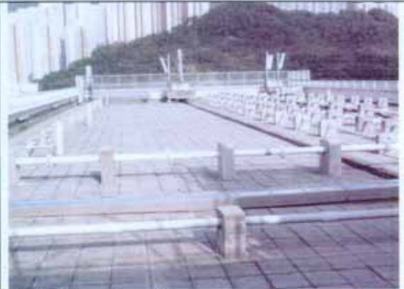
Vent pipes At roof
