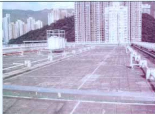
Vent pipes at roof
