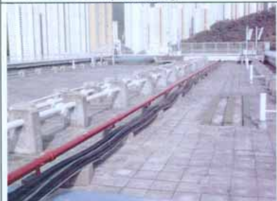
Vent pipes at roof
