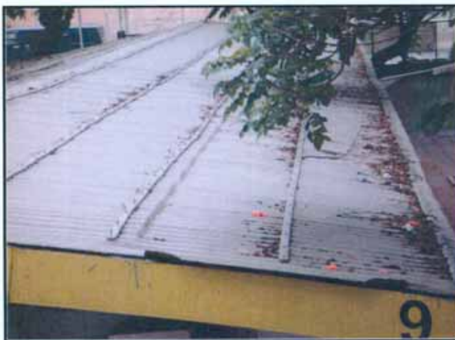
3. DESCRIPTION : Asbestos corrugated sheet at roof of blk. 9
