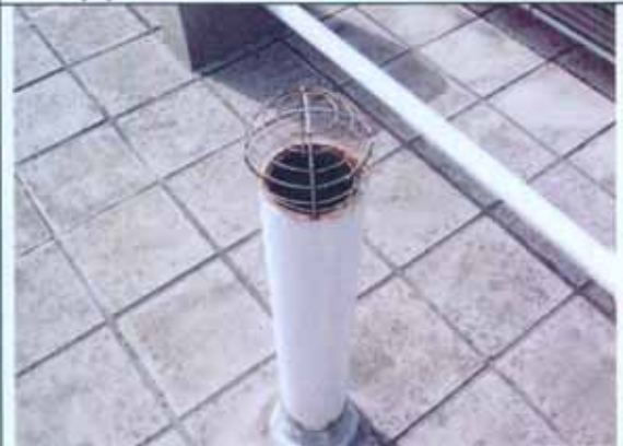
Condition of vent pipe
