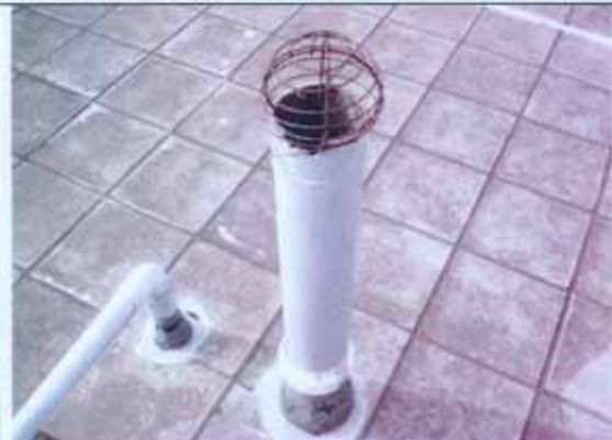
Condition of vent pipe
