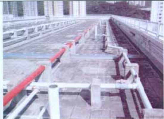
Vent pipes at roof
