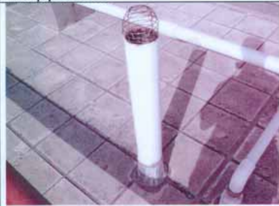
Condition of vent pipe
