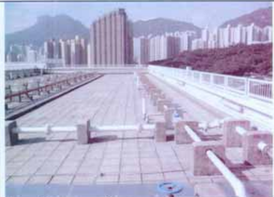
Vent pipes at roof
