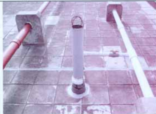
Condition of vent pipe
