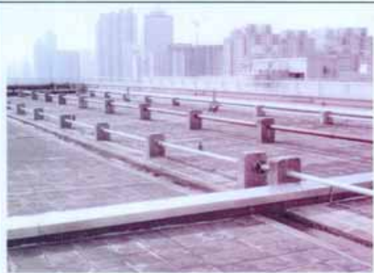
Vent pipes at roof
