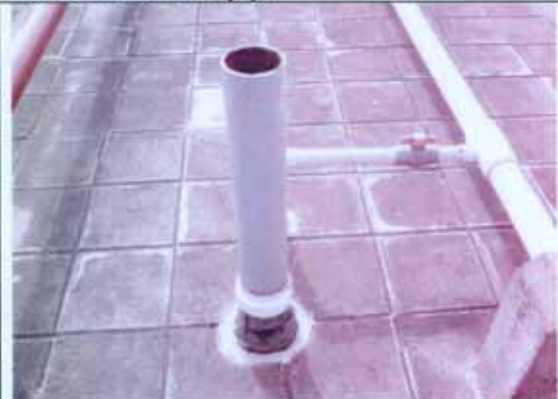
Condition of vent pipe
