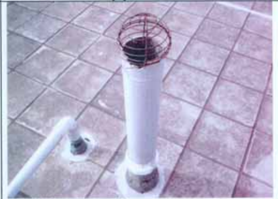
Condition of vent pipe
