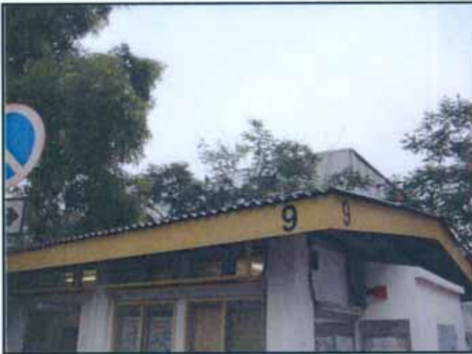
1. DESCRIPTION : Asbestos corrugated sheet at roof of blk. 9
