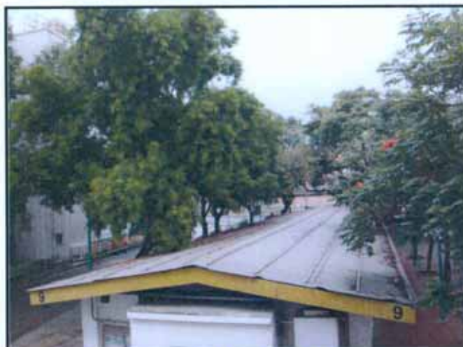
5. DESCRIPTION : Asbestos corrugated sheet at roof of blk. 9
