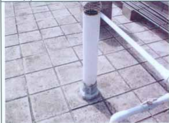
Condition of vent pipe
