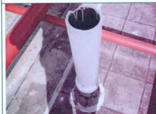
Condition of vent pipe
