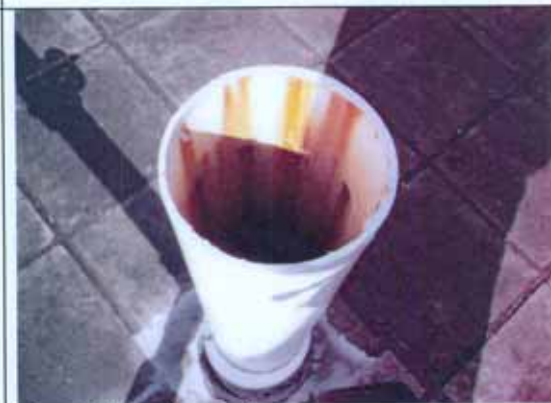
Condition of vent pipe
