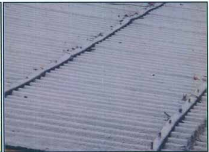
4. DESCRIPTION : Asbestos corrugated sheet at roof of blk. 9
