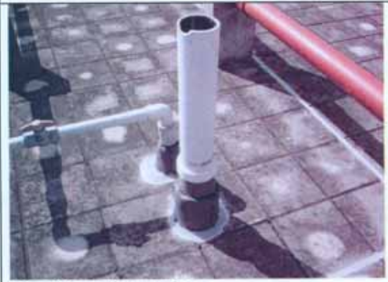
Condition of vent pipe
