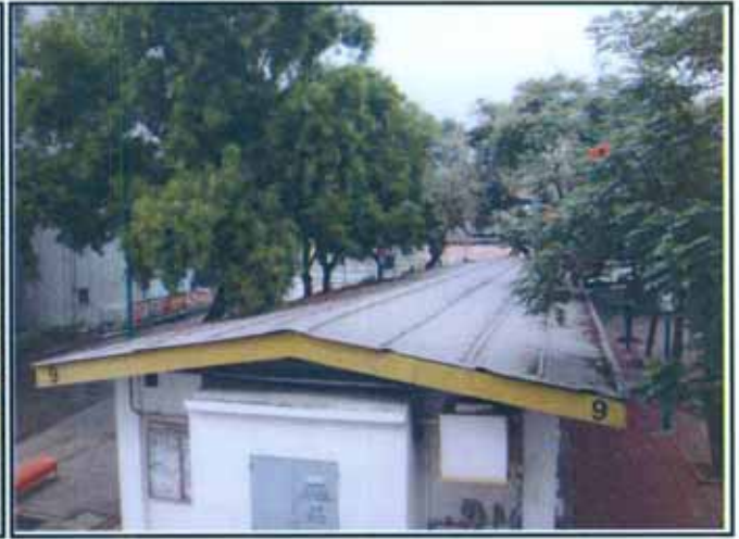
2. DESCRIPTION : Asbestos corrugated sheet at roof of blk. 9
