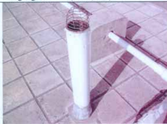
Condition of vent pipe
