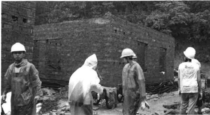
Construction site of the 2012 Habitat for Humanity Asia-Pacific Youth BUILD in Shuiweidong Village, Conghua, Guangdong, China. Photo: Hongyu Wang
