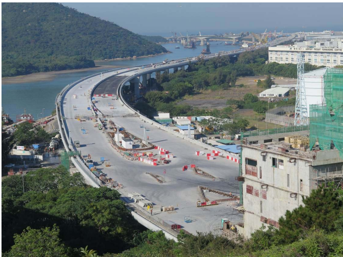
Figure 10: Installation of bridge decks of the land viaduct of the HKLR was completed. Bridge deck surfacing works are in progress.
