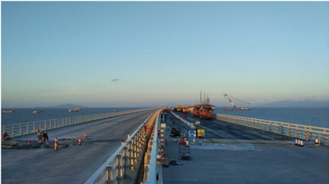
Figure 2: Installation of bridge decks of the HZMB Main Bridge was completed. Bridge deck surfacing works are in progress.
