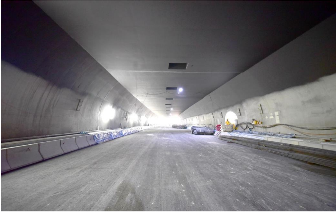
Figure 11: Construction of the Scenic Hill Tunnel of the HKLR is in progress.
