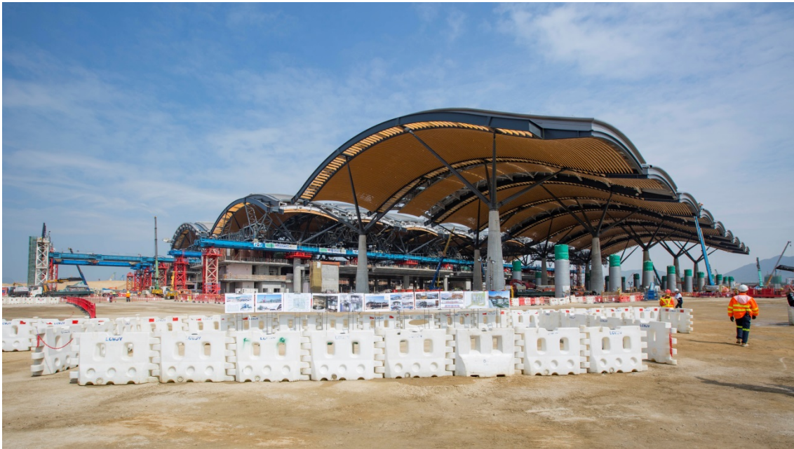
Figure 5: Installation of prefabricated roof segments for the Passenger Clearance Building of the HKBCF is in progress.
