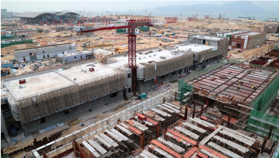
Figure 7: Construction of ancillary buildings and associated facilities of the HKBCF is in progress.
