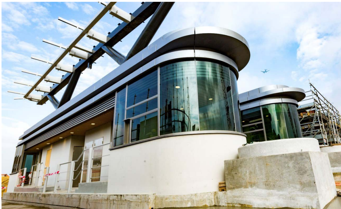
Figure 6: Construction of kiosks at the Vehicle Clearance Plaza of the HKBCF is in progress.
