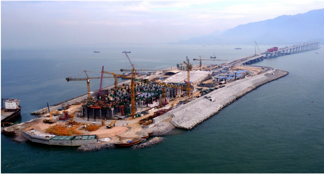
Figure 4: Construction of superstructures at the East Artificial Island of the HZMB Main Bridge is in progress.
