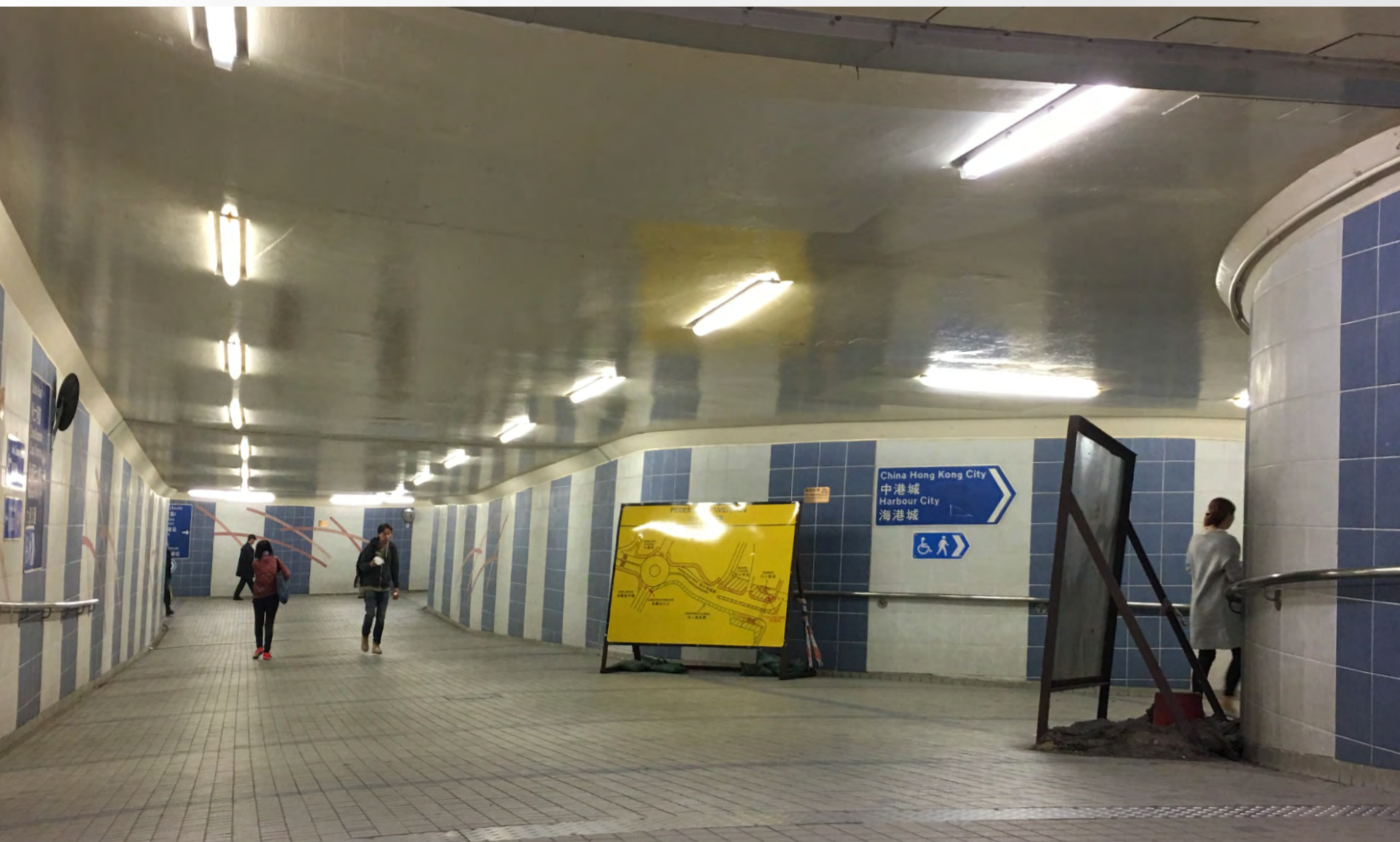
Interior of Austin Road Pedestrian Subway – Existing Condition 柯士甸道行人隧道內-現時狀況
