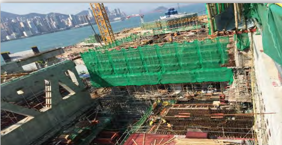
3/F slab at Zone F (roof terrace) F區的3樓板層 (頂樓平台)
