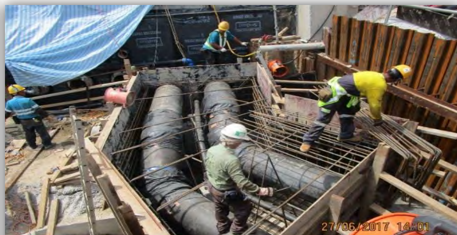
District Cooling System intake pipe (outside DCS Plant Room) 區域製冷系統進水管 (區域製冷機房外)
