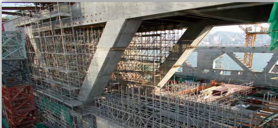
M/F wall, beam & slab construction between T1 & T2 T1 和 T2 桁架之間夾樓層建築
