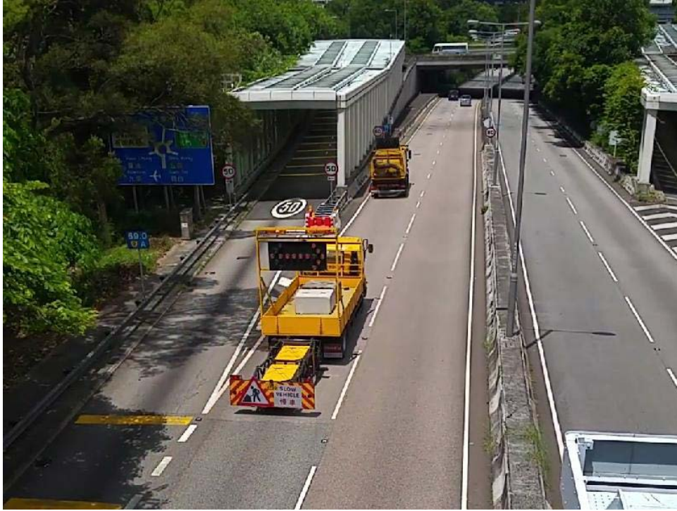
Figure 3: Escorted by a shadow vehicle with truck-mounted attenuator when conducting mobile operations
