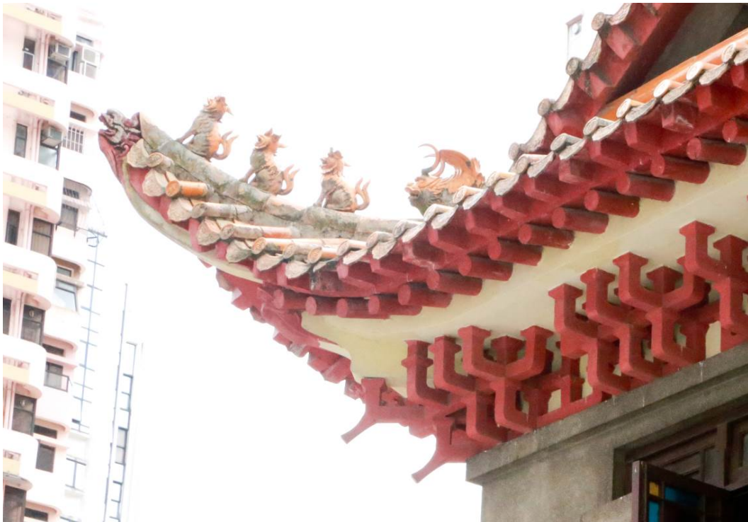
A set of ceramic running animals on a projecting eave. Decorative Chinese bracket sets under the eaves along roof edges.
