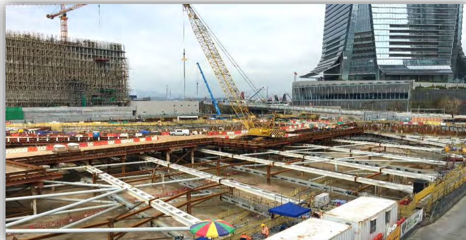
2nd layer strutting completed at northeast portion 完成東北間部分第二層支撐工程
