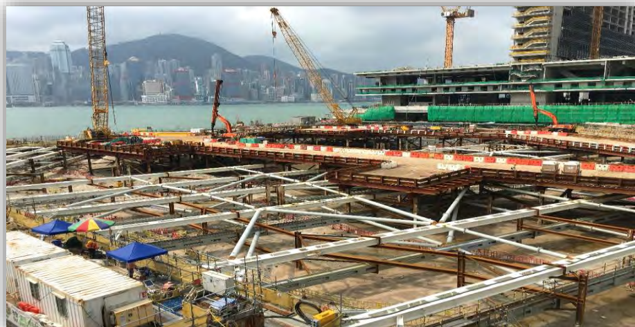
2nd layer strutting completed at middle portion (west) 完成中間部分第二層支撐工程
