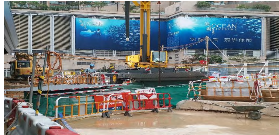
Portion 5 – Lifting Operation at ground level using reinforced concrete slab opening (Portion 5)
