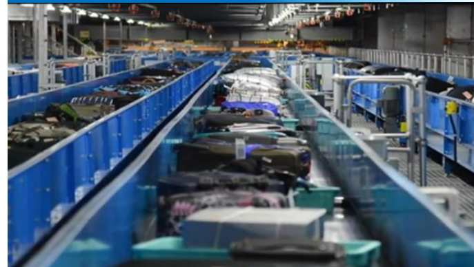
Predictive Maintenance for Baggage System
